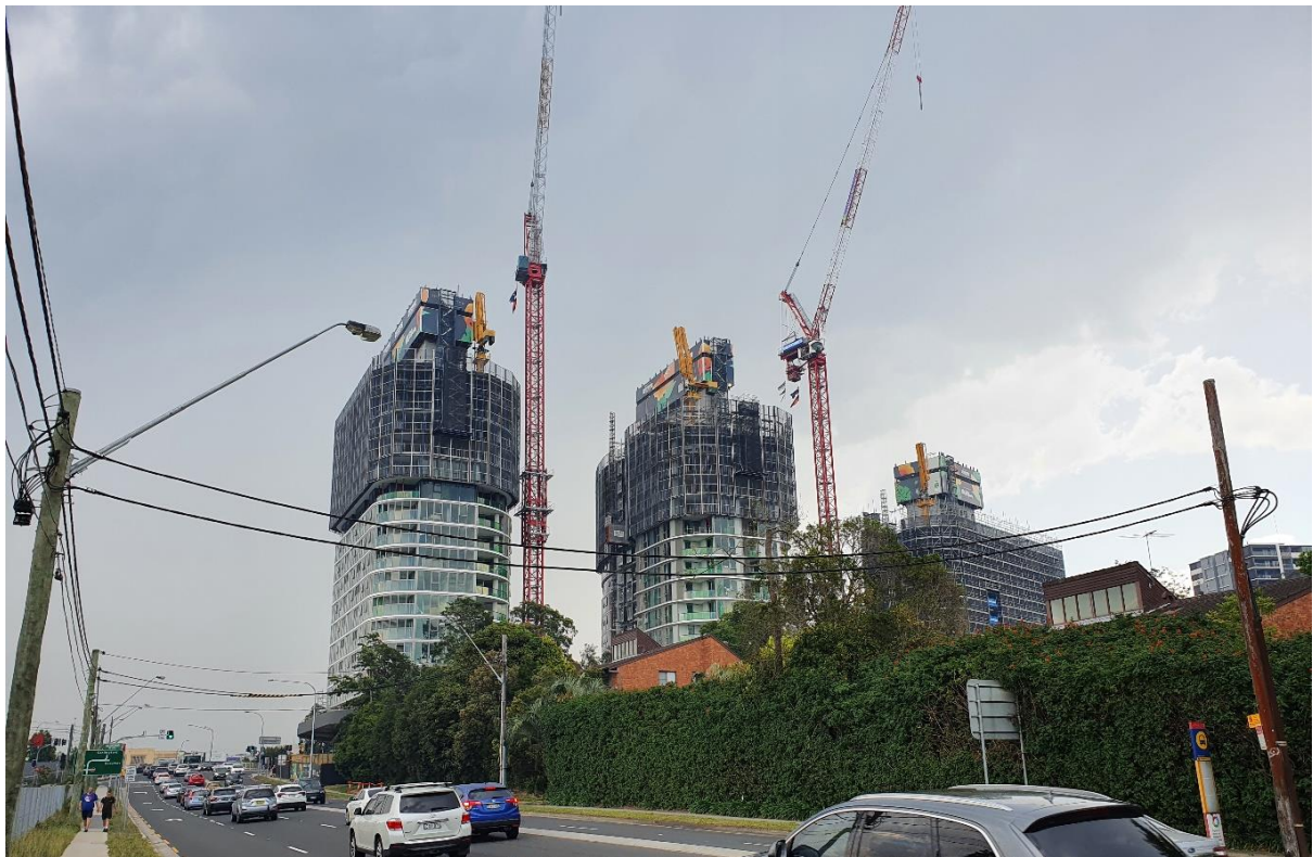
Figure 14: Three towers forming part of No. 12-22 Langston Place currently under construction, viewed from Epping Road to the east
